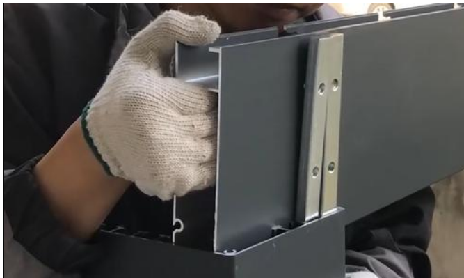
7. Put the connecting block on the beam into the slot of the column.
