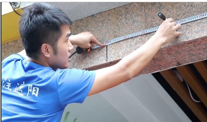
7. Measure the distance of the wall yard and mark it with a marker
