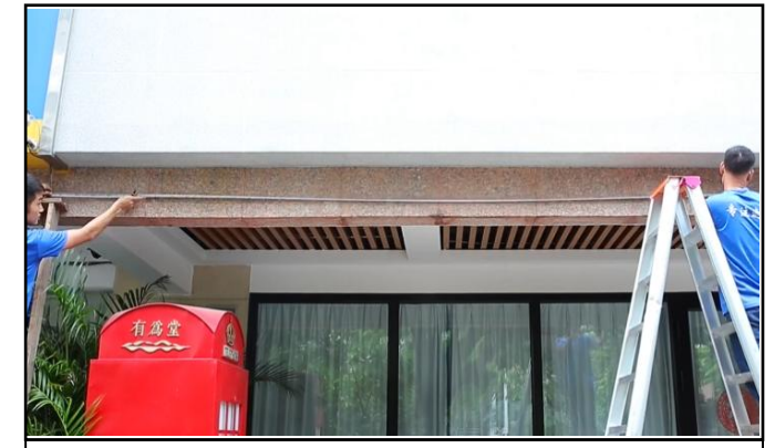
6. Confirm the installation position and distance on the wall according to the data just measured
