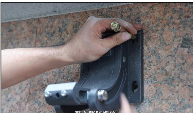
10, knock in the expansion screw, pay attention to keep the wall yard horizontal installation and distance from the top wall. Tighten the screws.
